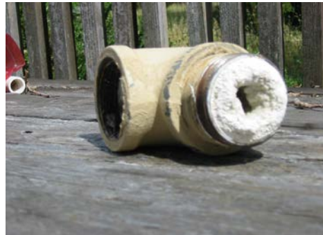
Figure 6. Struvite ( \text{MgNH}_4\text{PO}_4 \cdot 6\text{H}_2\text{O} ) is a source of P and N and can cause blockages in sewer pipes.
