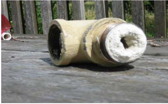
Figure 6. Struvite ( \text{MgNH}_4\text{PO}_4 \cdot 6\text{H}_2\text{O} ) is a source of P and N and can cause blockages in sewer pipes. [After D. Merrill]
